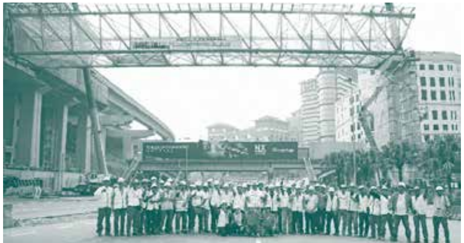
Installation of The Phileo Damansara MRT Station Link Bridge: The Largest Lifting Operation
