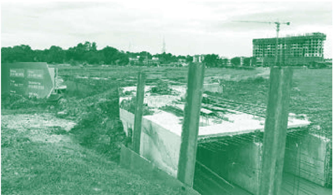
Proposed Flood mitigation project at Batu Lintang area, Kuching (2.5m wide box culvert at Jalan Rock (casted))
